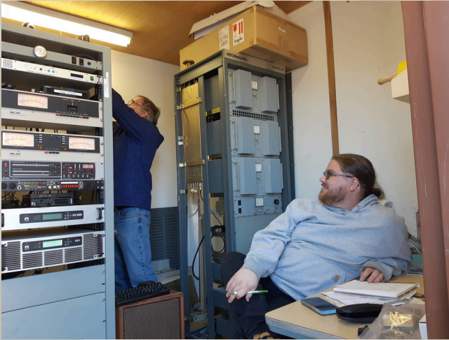
Eric Heidendahl (L) and Chancelor Maracle (R) inside CFRC's transmitter shack at our tower site.
